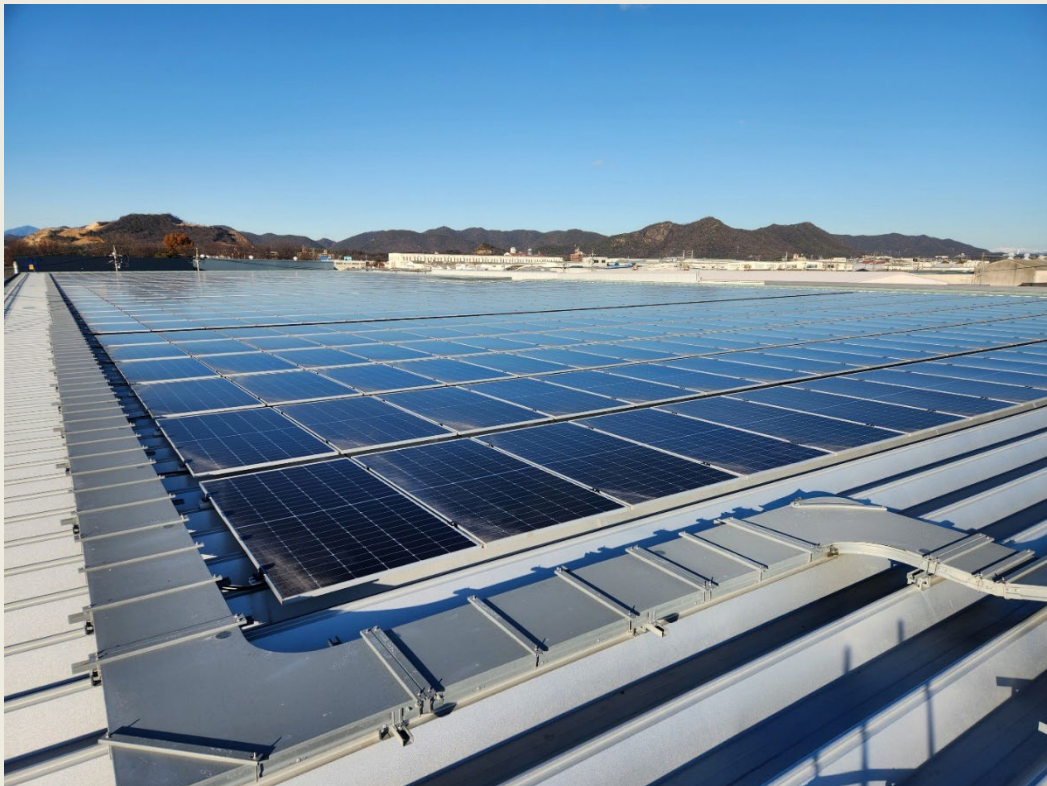
Gifu New Plant No. 1 Rated output: 437.5 kW Panel capacity: 550 W Number of panels: 894
